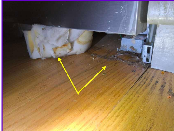
A minor leak was observed beneath the dishwasher.
