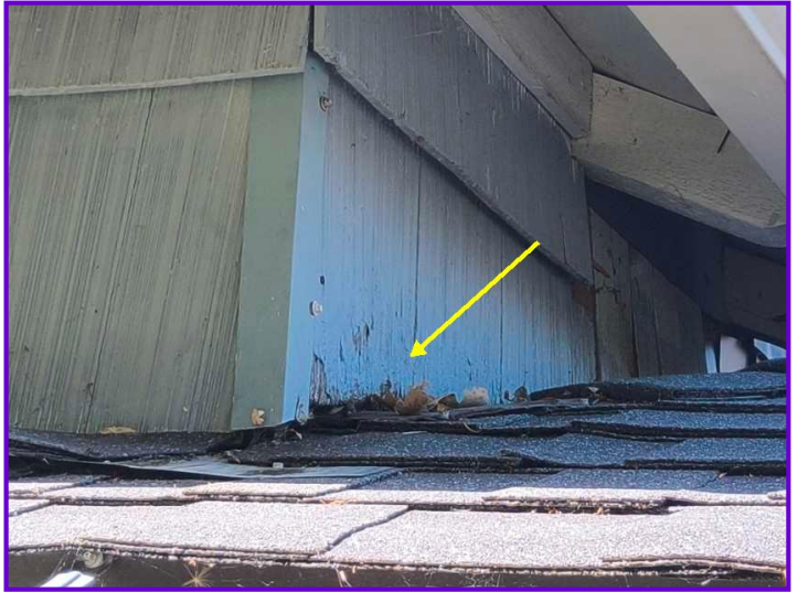
Gaps or openings were observed in the wall coverings.
