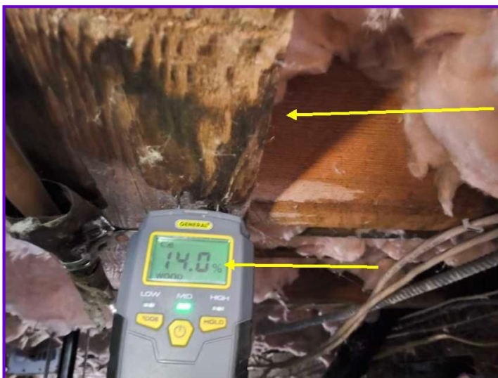
Moisture meter readings indicated slightly elevated moisture levels consistent with the leak observed under the dishwasher.
