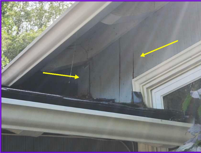
Gaps or openings were observed in the wall coverings.
