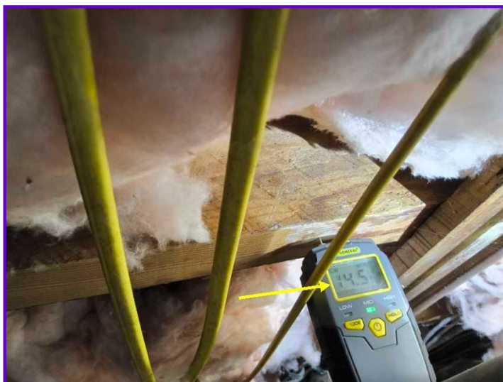
Moisture meter readings indicated slightly elevated moisture levels consistent with the leak observed under the dishwasher.
