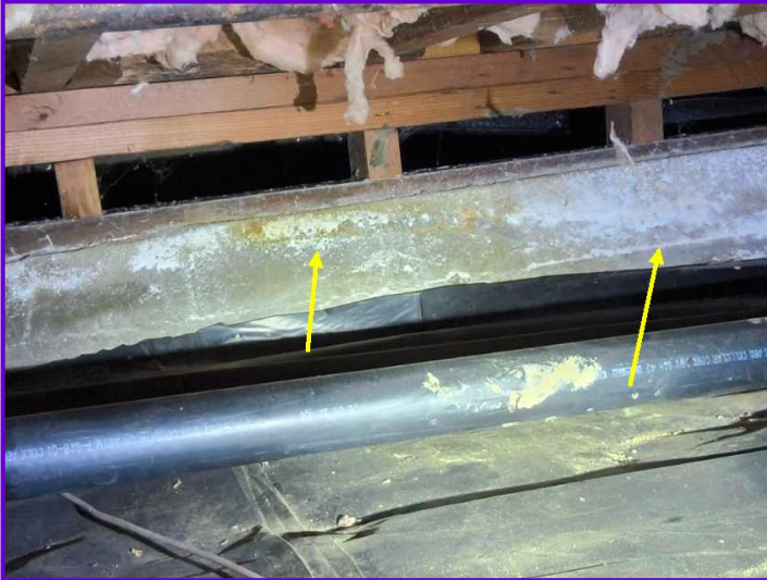
Efflorescence was observed at the concrete raised foundation walls.
