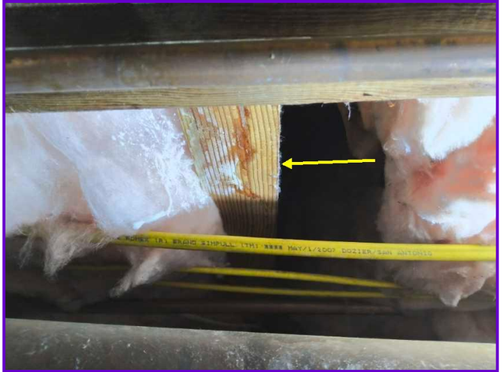
Water staining was observed on the subfloor beneath the kitchen area.
