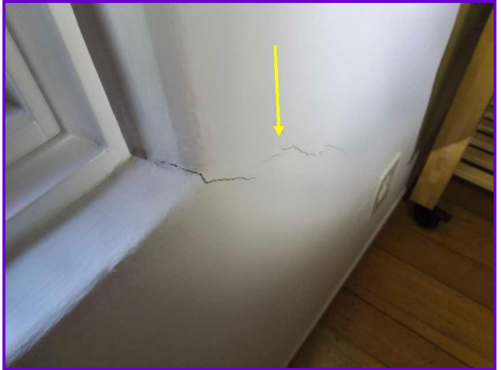
Minor cracks and bubbling in the wall finish were observed.
