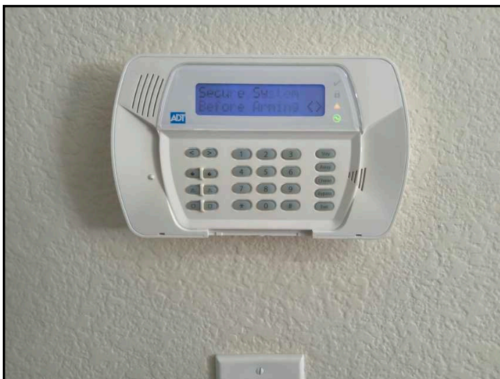
WI-FI SECURITY SYSTEM – NOT INSPECTED: The property is equipped with a removable Wi-Fi camera/security system.
