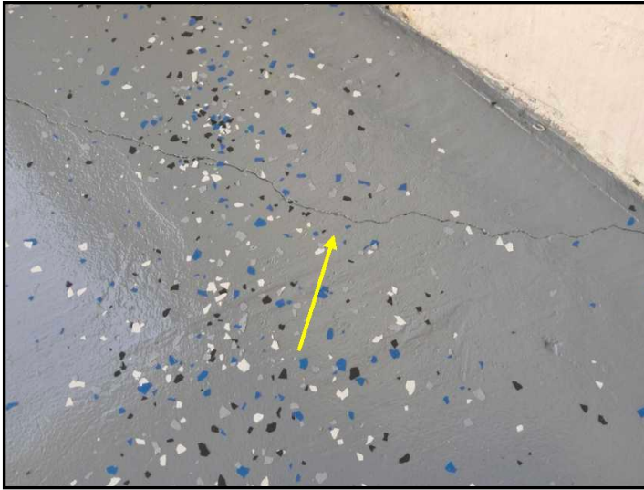
COMMON CONCRETE CRACKS: Common cracks were observed in the garage slab.
