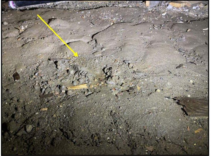
An active leak was observed from the potable water supply piping.
