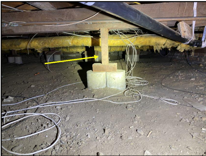
Unconventional supplemental supports were observed beneath the older section of the house.
