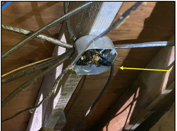
Open electrical box was noted during the inspection.
