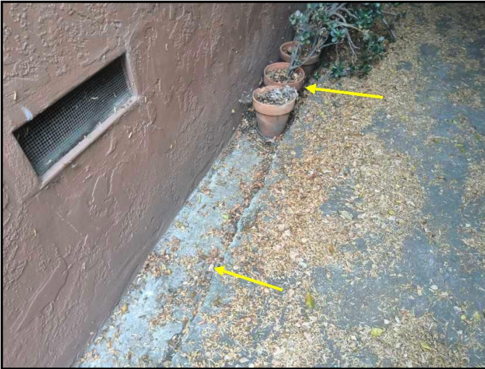
A gap was left between the concrete sidewalk and the foundation when the new foundation was constructed.
