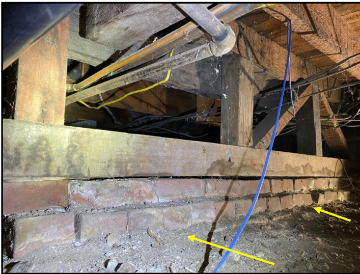
One or more supplemental foundation support walls were constructed with unreinforced mortared brick.
