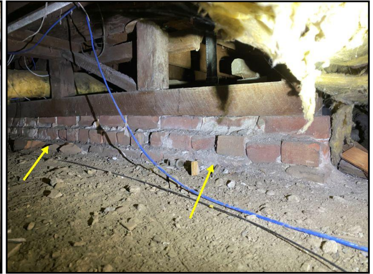
One or more supplemental foundation support walls were constructed with unreinforced mortared brick.
