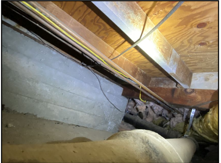
There are areas under the property that are not insulated.
