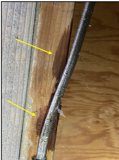
Visible evidence of an active water leak was observed dripping from the subfloor.
