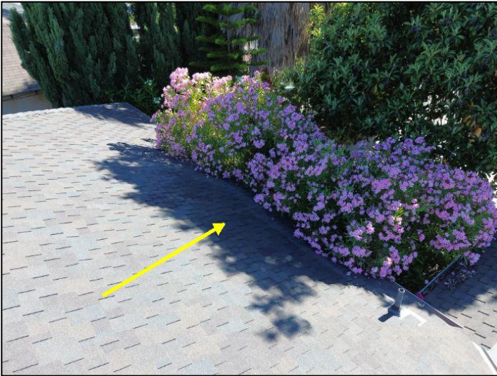
FOLIAGE NOTED: Foliage was observed growing over or in proximity to the roof.
