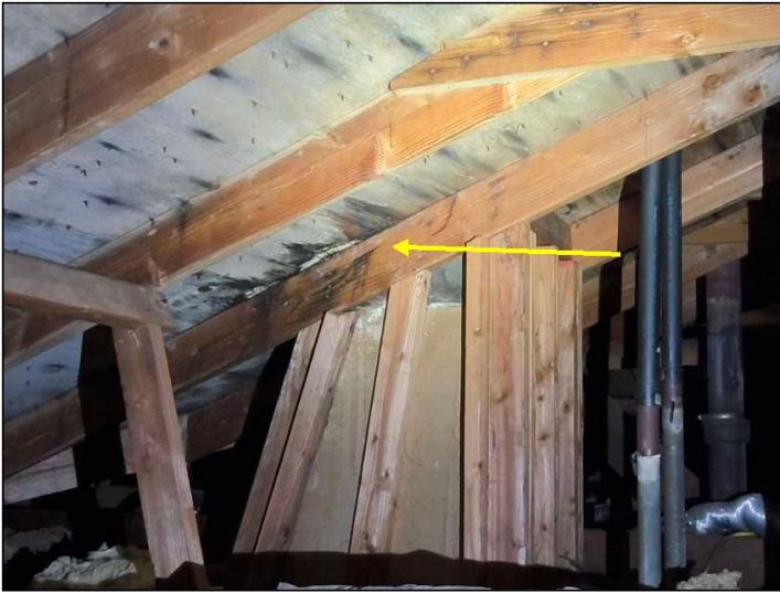
Moisture stains were observed on the attic framing and sheathing.
