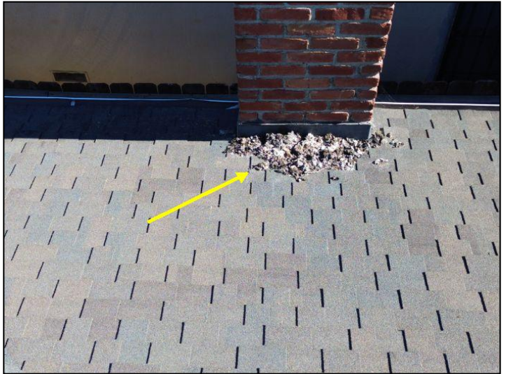
DEBRIS ON THE ROOF: Leaves and debris were observed in portions of the roof near the chimney.
