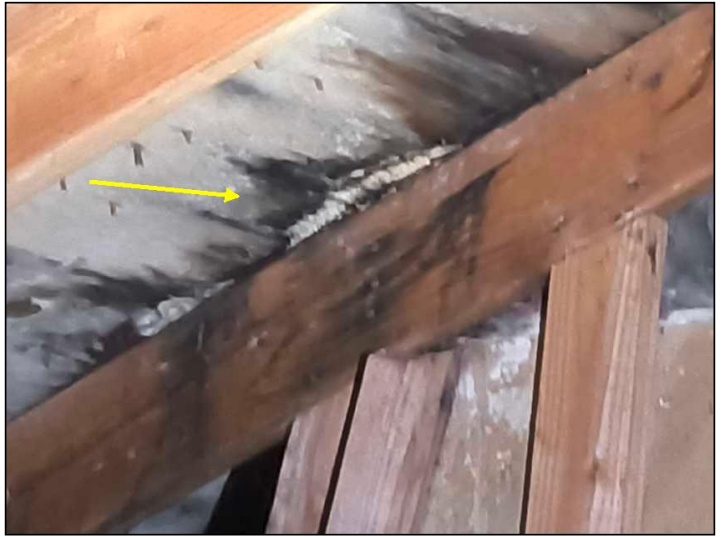
The staining near the skylight appeared consistent with an active leak at the time of the inspection.
