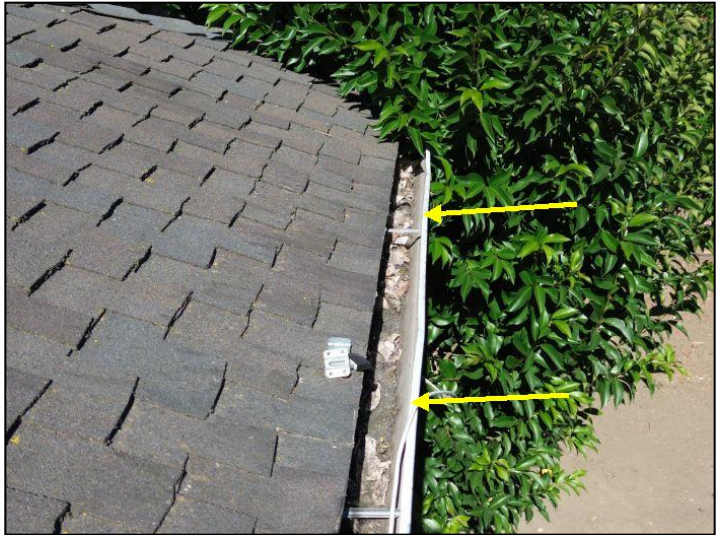
The roof gutters require cleaning to function effectively.
