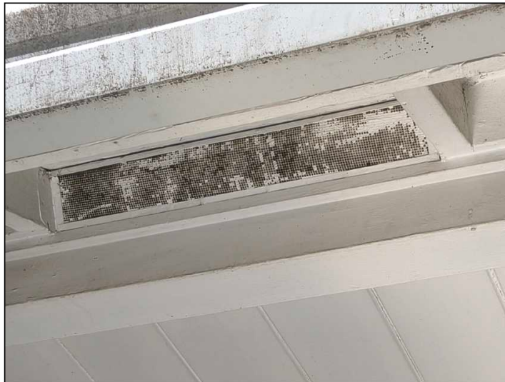
Vent screens noted painted over.
