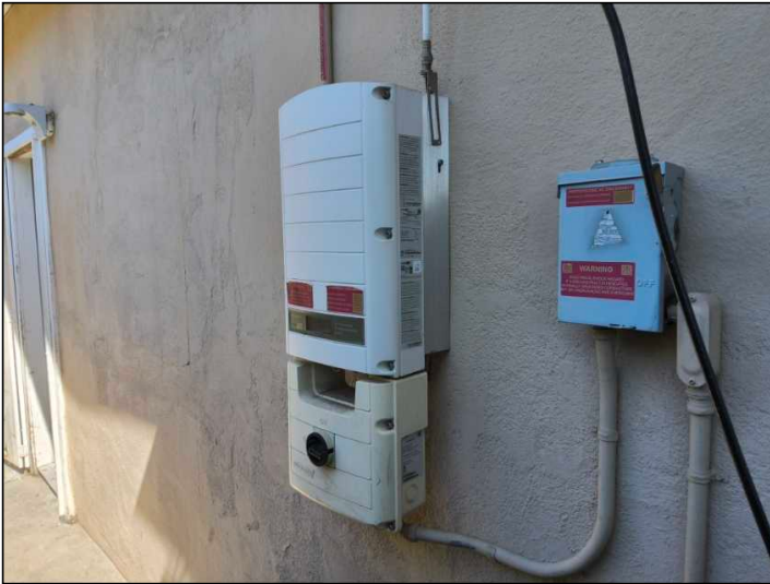
The roof is equipped with photovoltaic (solar) panels.
