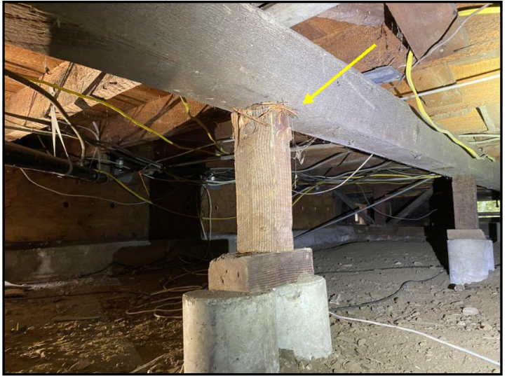
Conditions included amateur installation, the use of 2x4 wood members without proper brackets or mechanical connections.
