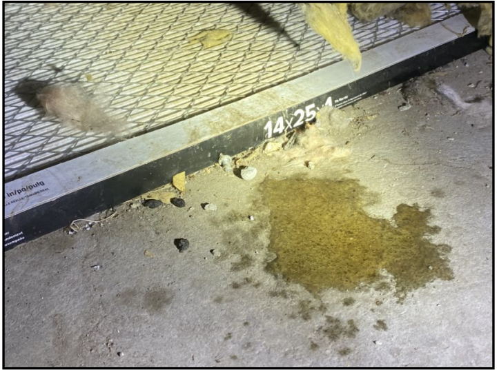
Visible evidence of an active water leak was observed dripping from the subfloor.
