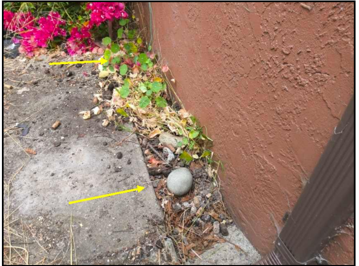
Water can collect and remain within this space, allowing prolonged moisture exposure against the foundation stem wall.
