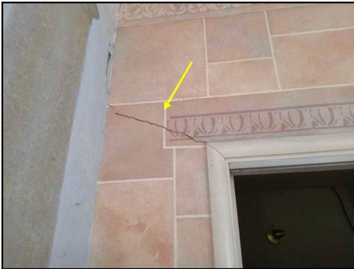
Minor drywall separation and cracking were observed at the walls.
