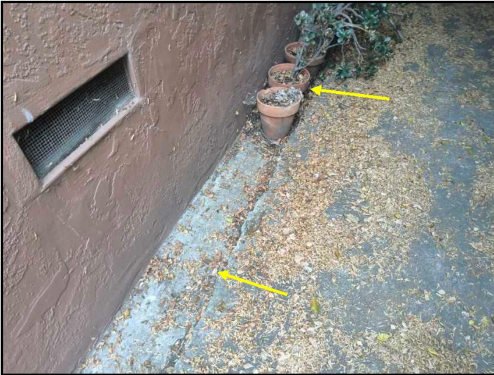
A gap was left between the concrete sidewalk and the foundation when the new foundation was constructed.
