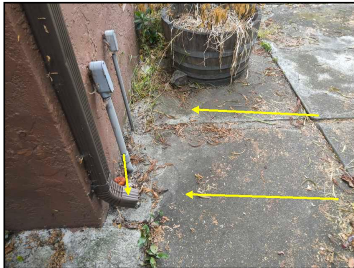
GRADING AGAINST FOUNDATION: The exterior grading is improperly sloped towards the foundation.
