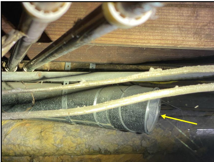
A section of the forced-air heating duct system in the crawlspace was observed to be disconnected or unattached.
