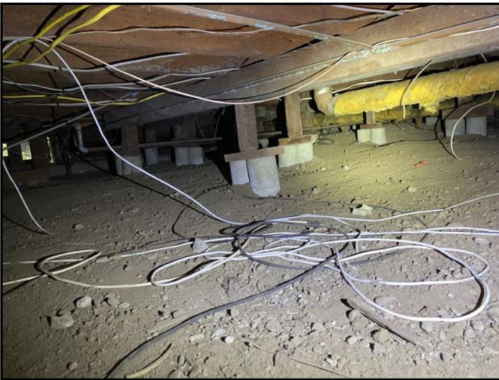
Unconventional supplemental supports were observed beneath the older section of the house.
