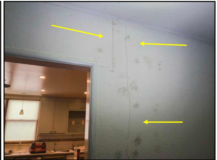
Minor drywall separation and cracking were observed at the walls.
