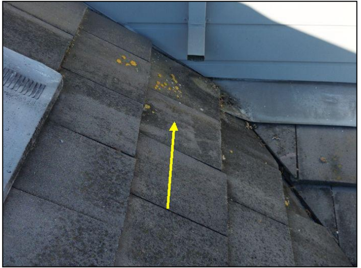
ROOF-TILE CLEANING: Moss growth was observed on the roof tiles.
