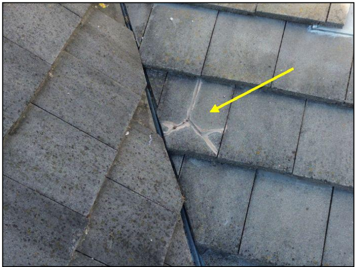
CRACKED TILES: One or more cracked roof tiles were observed.
