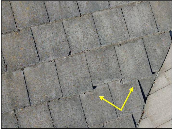
SLIPPED TILES: Some roof tiles, particularly near the valley flashing, were loose, displaced, or had slipped from their intended positions.
