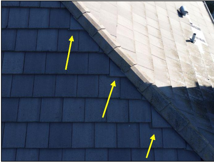
SLIPPED TILES: Some roof tiles were loose, displaced, or had slipped from their intended positions.
